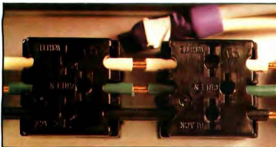
Photo 4: Using an X-acto knife or similar tool, strip insulation from the wires between the receptacles (which I number 1 through 4, from left to right) according to the following system: between 1 and 2, strip the green and black; between 2 and 3, strip the green and white; between 3 and 4, strip the black and white.
