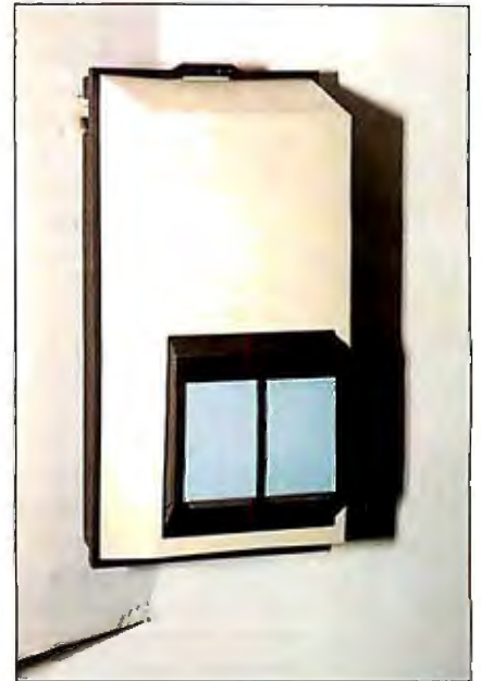
Photo 2: Much of my application for the HCS deals with its use for security and automatic lighting. Shown is the installation of a typical passive infrared motion detector. Costing in the neighborhood of $140 each, these units detect the movement of objects (like people) that have a different temperature than the surroundings. The units require a 12-V power source. Output is a contact closure: closed is no motion and open is motion detected.
